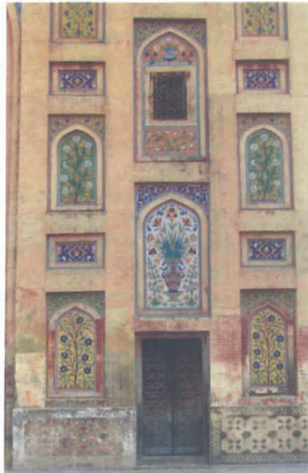
Figure 4: panels of the vestibule from the courtyard side showing Kashi-kari in sunken panels. The mid one is broader and larger panels
